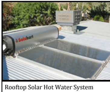
Rooftop Solar Hot Water System
