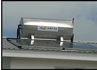
Rooftop Solar Hot Water System
